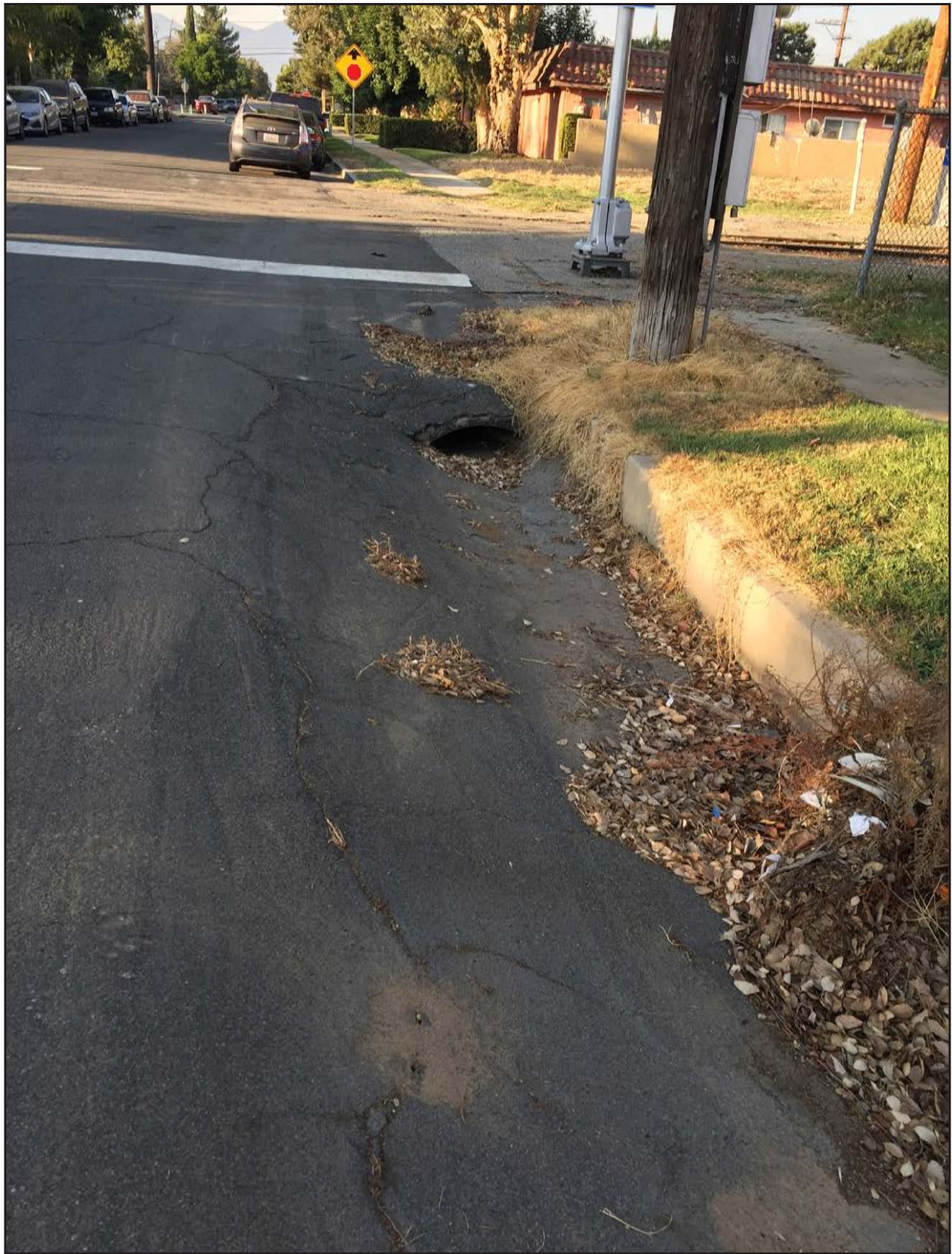
PHOTO 6e North Olive Ave - Drainagea
