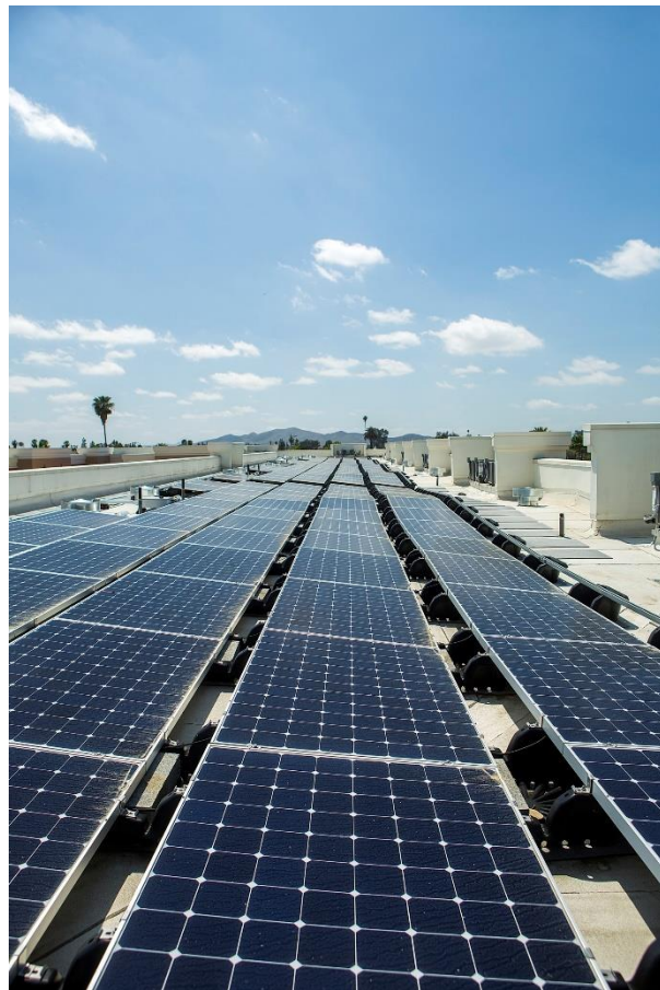
Example, Green Building Practice (Solar PV)
