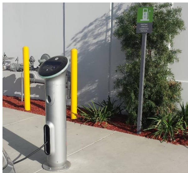
Example, Green Building Practice (EV Charging Station)
