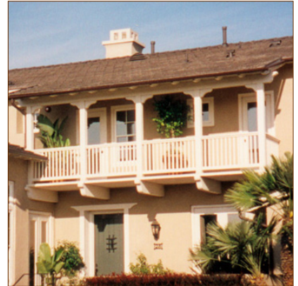
Exposed rafter tails
