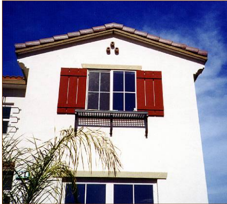
Little or no roof overhang at rakes
